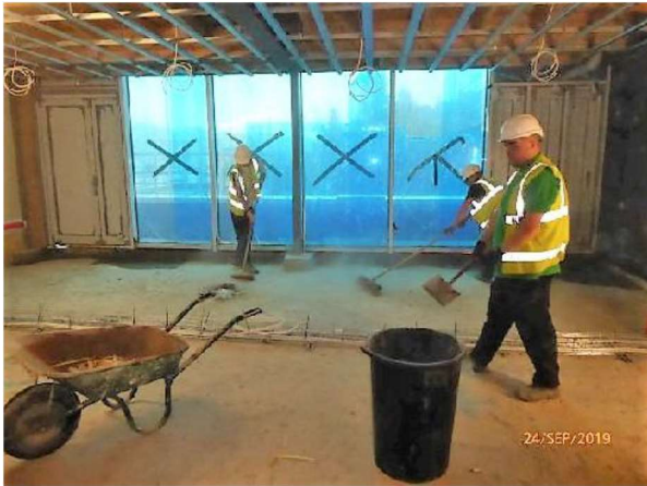
New Offices: Cleaning in progress in advance of suspended floor installation works.
