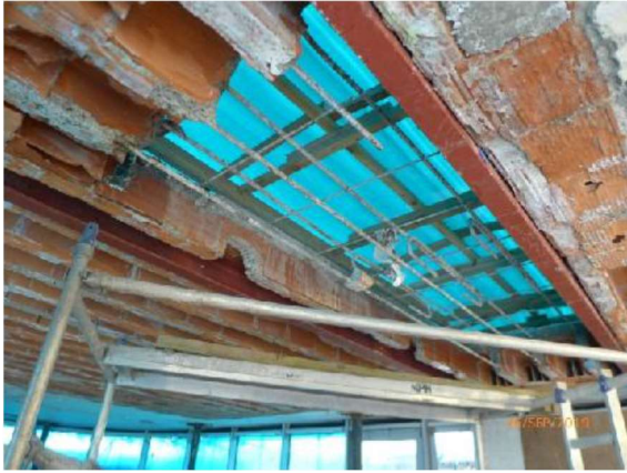
General View - Sections of the existing roof slab broken out to form the opening for the new AOV.
